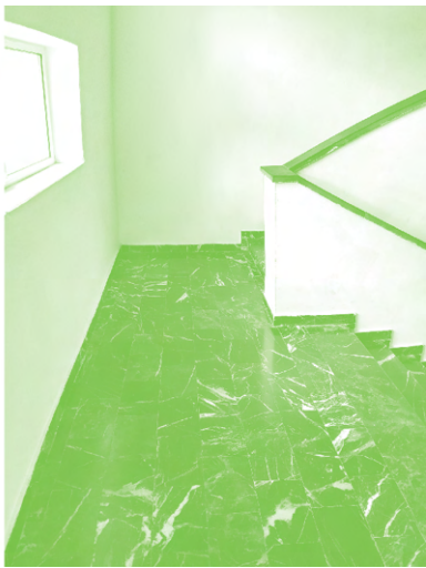
Fig. 9. Changes to the main staircase materials due to the 2004 reconstruction works, photo by Jora Kasapi CC BY-SA 4.0.
